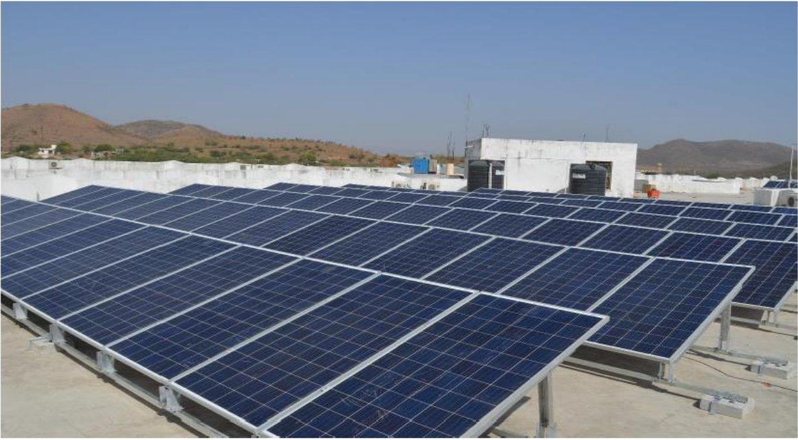
50 kW on grid Solar plant
