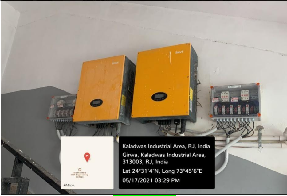
Solar UPS System
