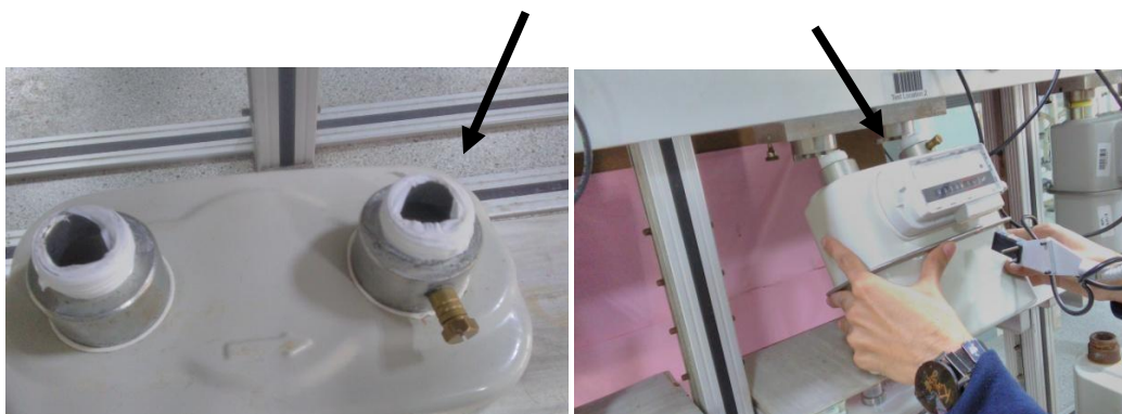
Figure 4.13: Software indicates the leak
