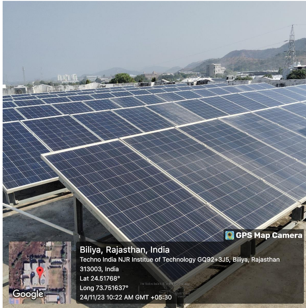
50 KW Solar Power Plant
