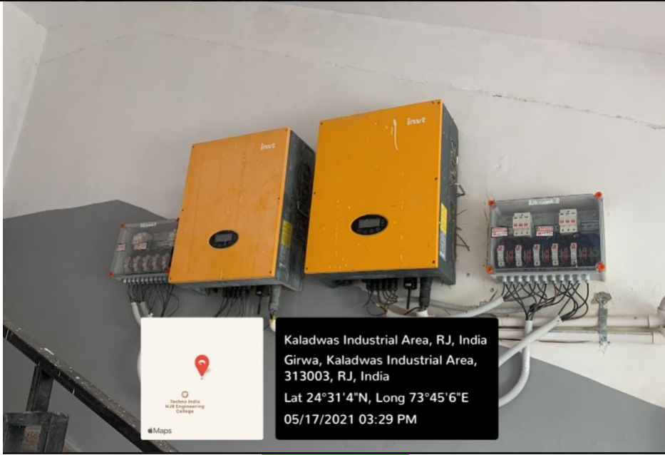
Solar UPS System
