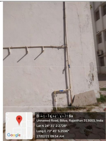
Supply to Bathrooms/ Toilets
