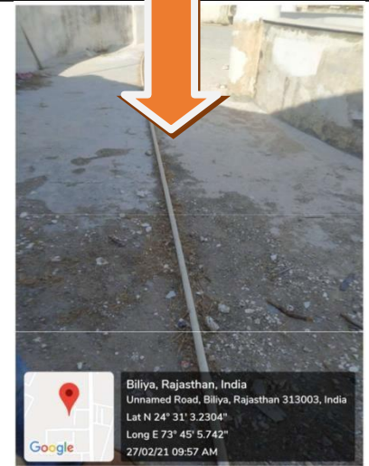
Line to RO on Roof
