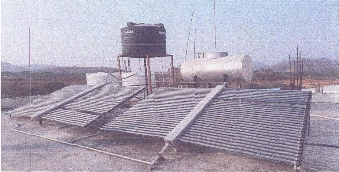
Solar Water Heater
