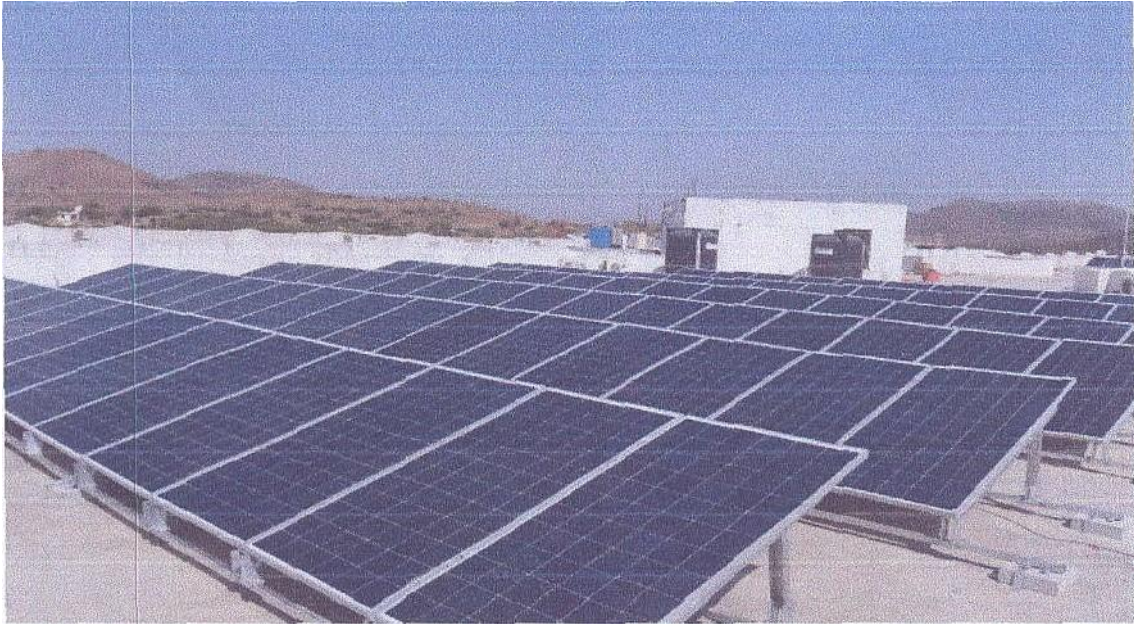
50 kW on grid Solar plant
