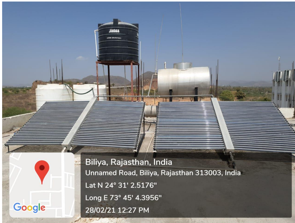
15. Solar Water Heater
